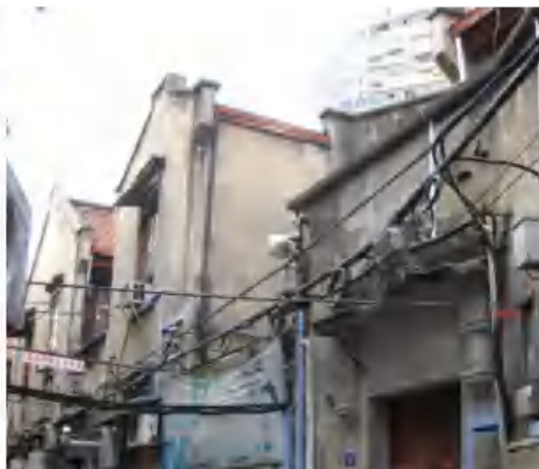
Figure 90: Cornice Parapet of Baoyuanli Before the Renovation
